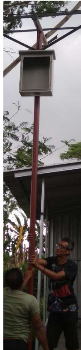
Figure 23. (right) Installation of An Evacuation Guiding Post. Photo: MRC
